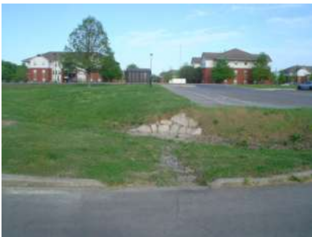
Figure 31: This shows the same area as figures as 29 and 30, yet this is on the other side of the inlet. The work done here was mostly for erosion control.
