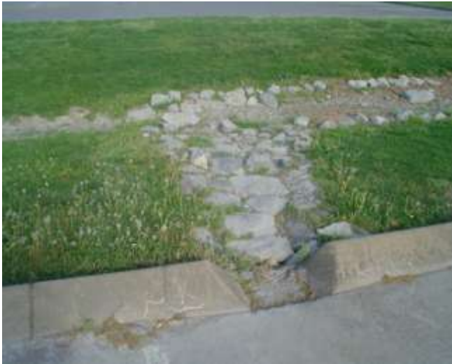
Figure 8: This is the same inlet shown in Figure 6 that flows from the parking lot into Raingarden #2.
