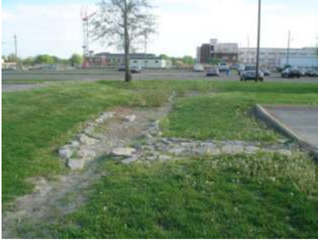
Figure 7: This is an inlet from a parking lot to Raingarden #2.
